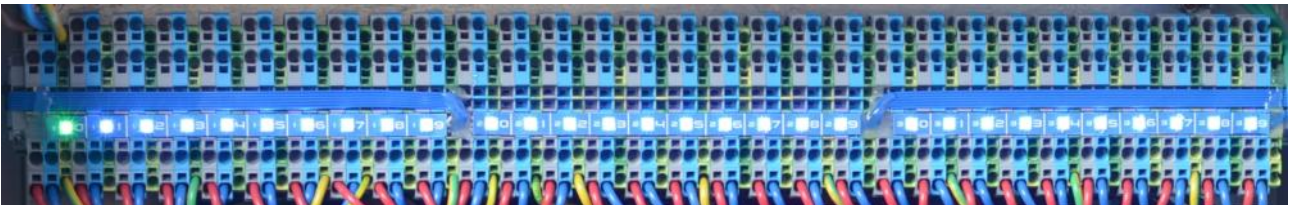
Figure 2.3.12. Upper panel with outlet terminal blocks as in case of RPCM 3x250.
