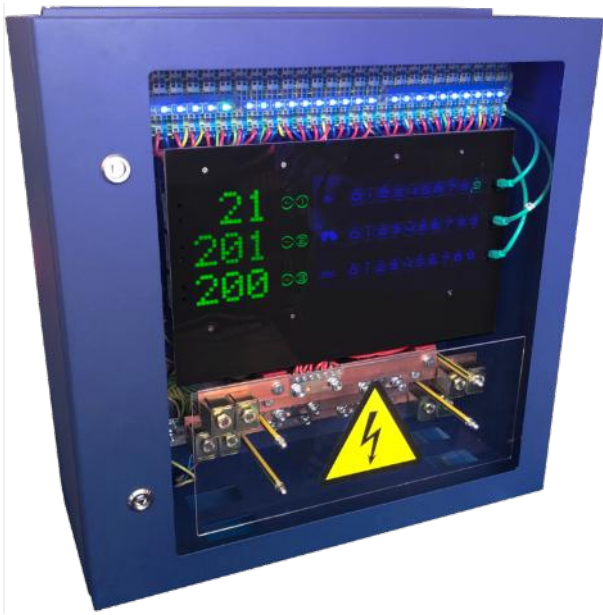
Figure 4.1.12. Appearance of RPCM 3x250 (the door is closed).
