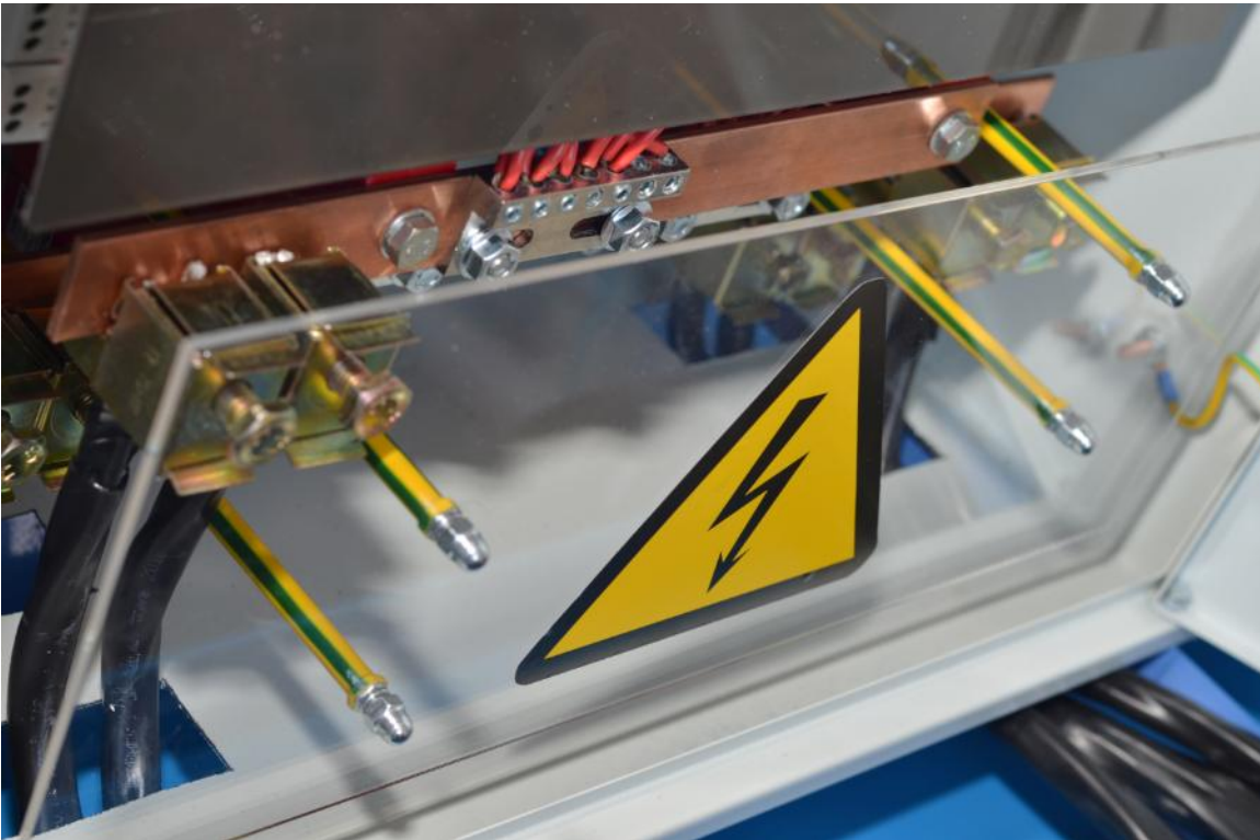
Figure 2.3.11. RPCM 3x250 with the insulating shield installed (white-gray background was pictured for more contrast).
