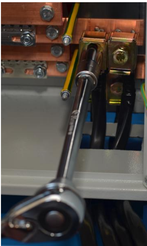
Figure 2.3.7. Connecting the cable to the terminals on the input (white-gray background was pictured for more contrast).
